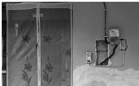
Figure 2 Uncanny aspects of public housing: Transformation of corridor into a hanging garden (top) and bypassing of utility (bottom) (Photographs by author)
